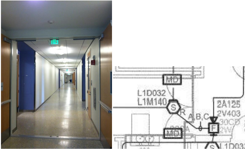
Figure 18 - Photo of magnetic door smoke detector and plan view [10].
