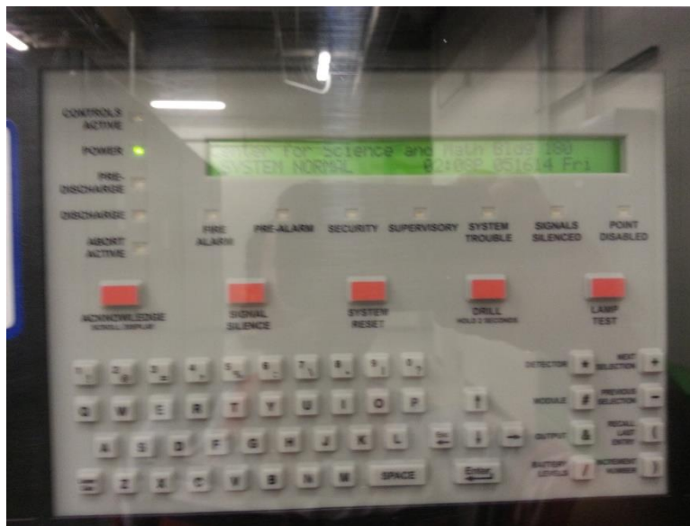
Figure 13 - Honeywell Notifier fire alarm control panel.
