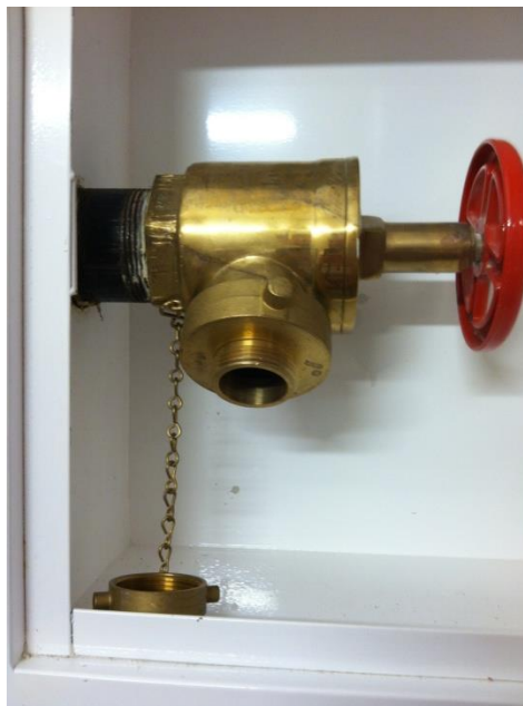
Figure 9- Standpipe hose connection with 2 1/2" and 1 1/2" connections.
