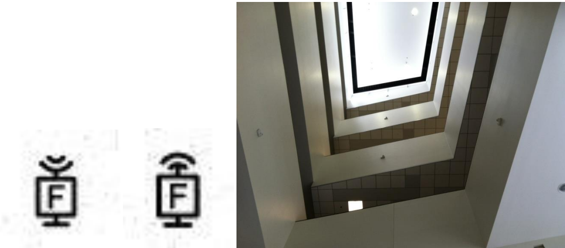
Figure 20 - Plan symbol of beam detector receiver, imager, and photo of beam detectors in atrium.
