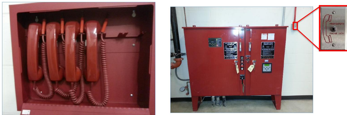
Figure 11 –Telephones jack and portable handsets located at fire pump room
