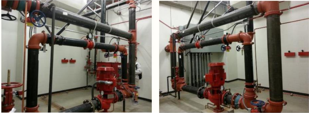
Figure 48 – Equipment in the Fire Pump Room
