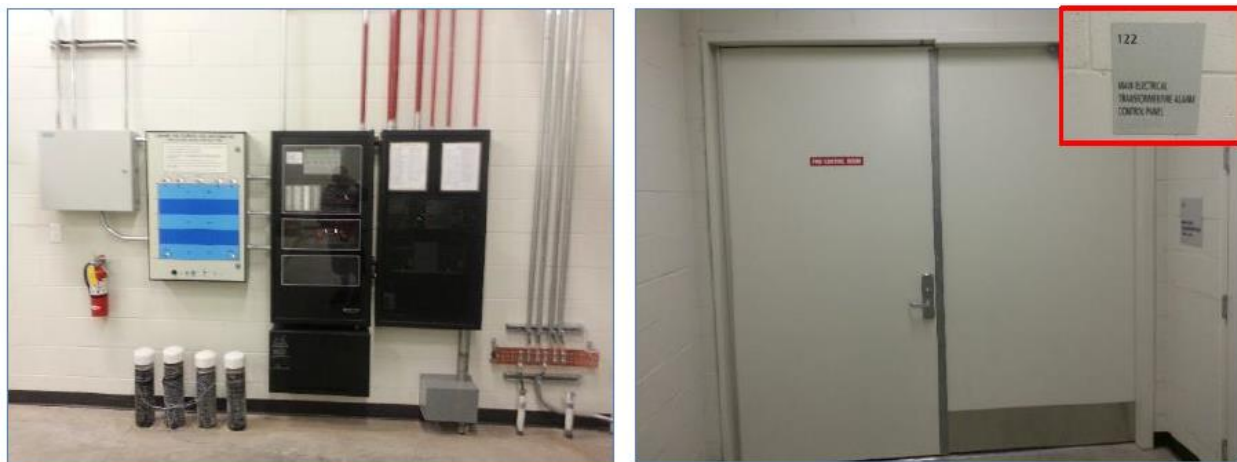
Figure 10 – FACU installed in CSM, Room 122
