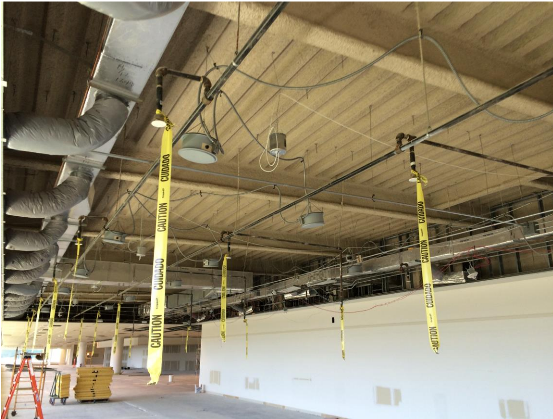
Figure 52 Sprinkler System Left In Service During Construction
