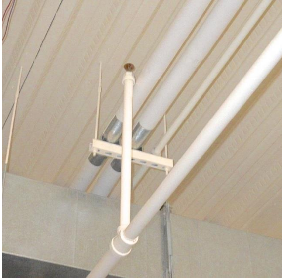
Figure 24 Sprinkler Obstructed by Mechanical Piping
