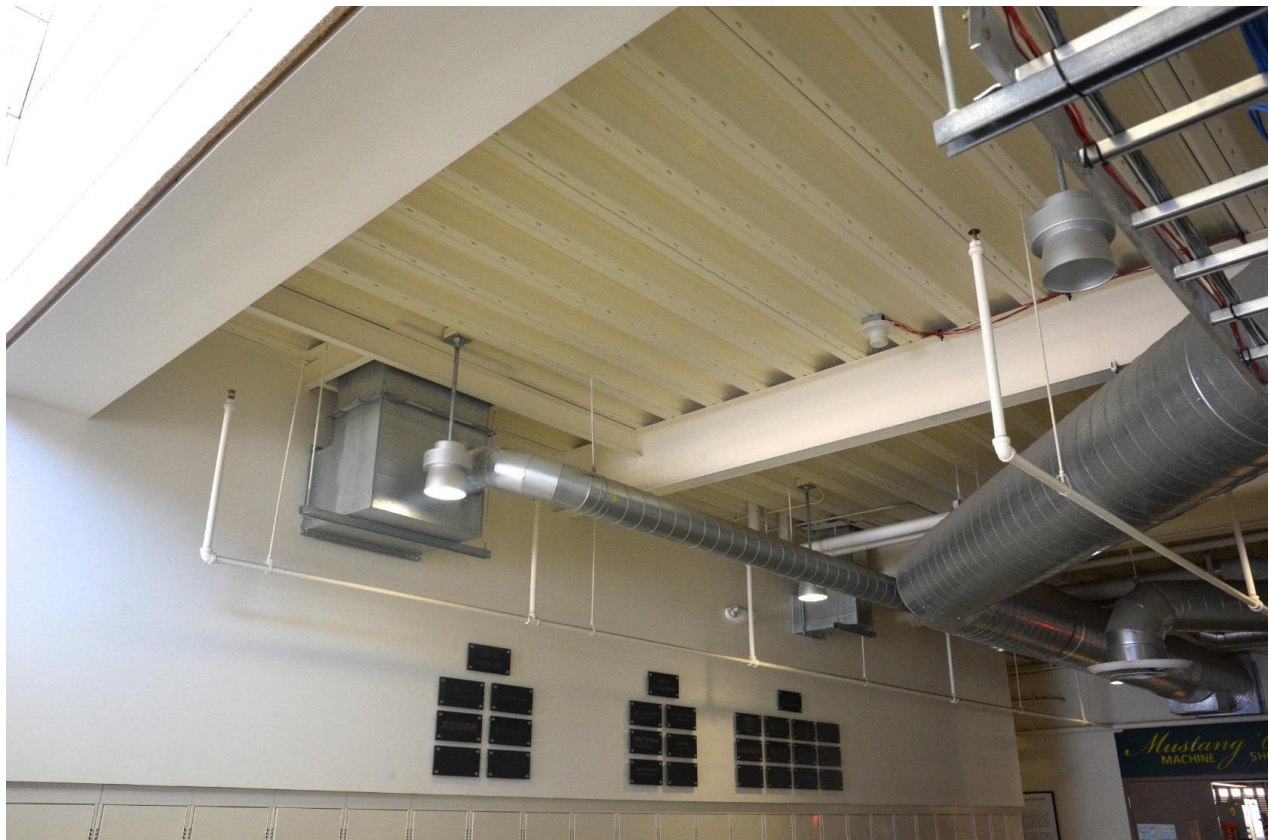
Figure 23 Branch Lines Missing End of Line Restraints
