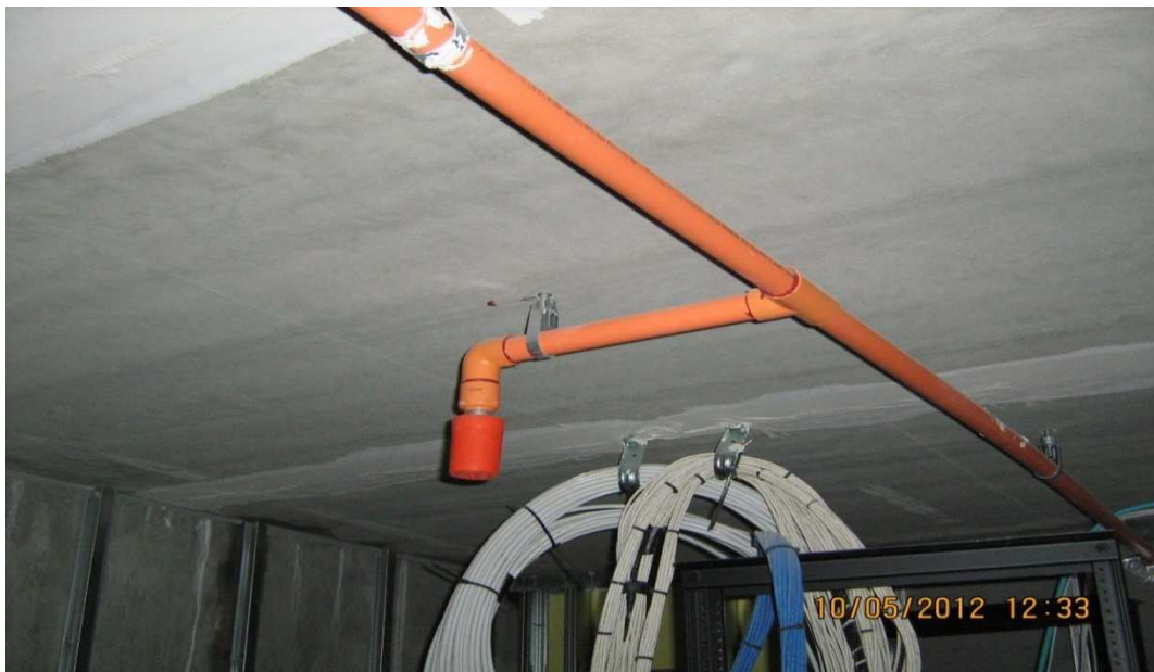
Figure-26: Sprinkler Pipe Photo II
