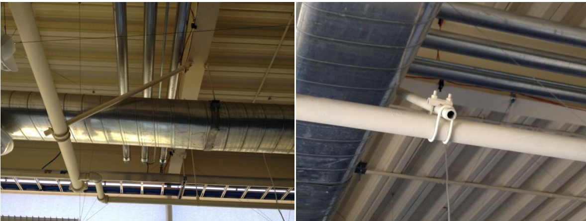
Figure 17: Example of Fire Sprinkler Bracing
