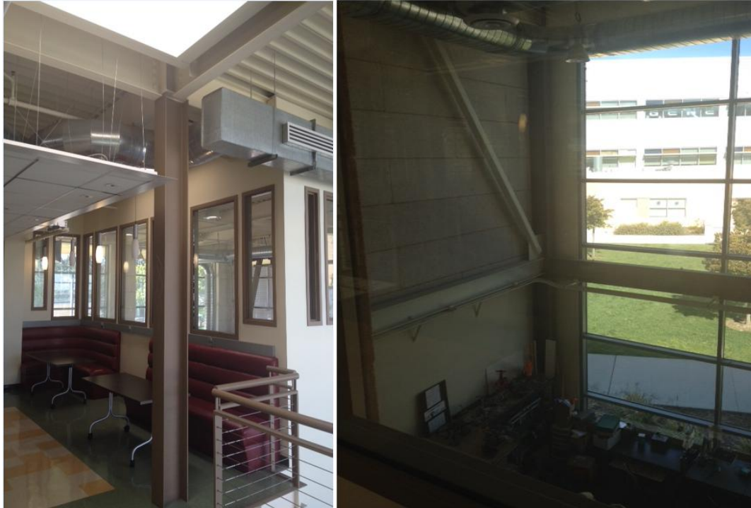
Figure 5: Unprotected/Exposed Structural Columns – 0 hr Fire Resistance Rating
