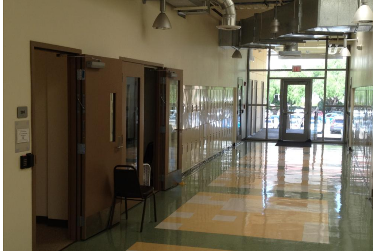
Figure 23: Interior Doors Propped Open
