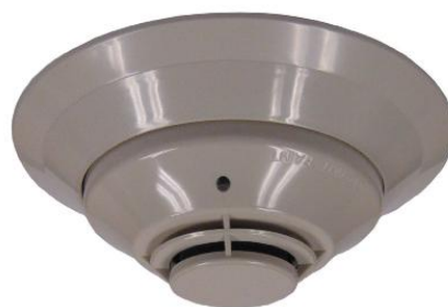
Figure 8: Notifier (FST-851) Heat Detector
