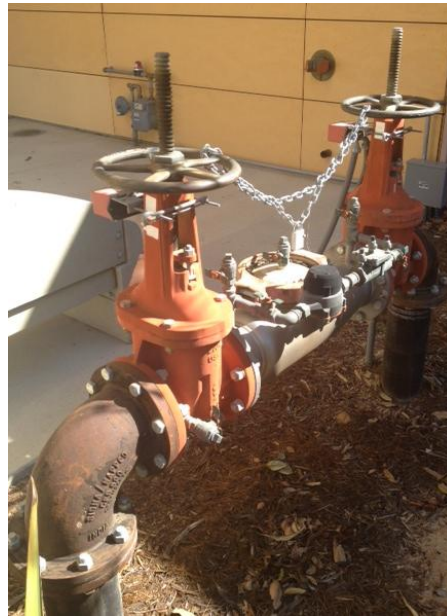
Figure 13: Fire Department Connection and Double Back Flow Preventer
