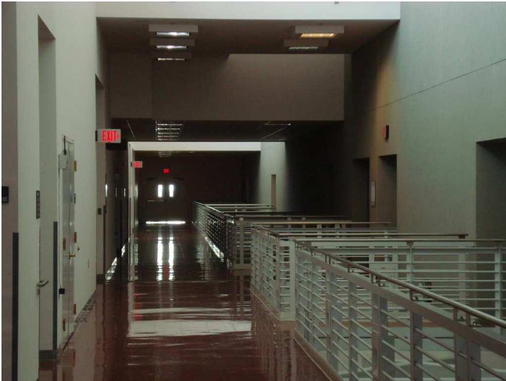
Figure 5-3. RMSEL exit signs
