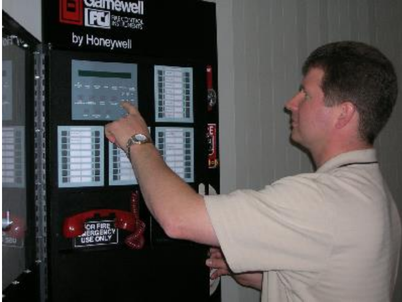
Figure 3.2: Fire alarm system maintenance works
