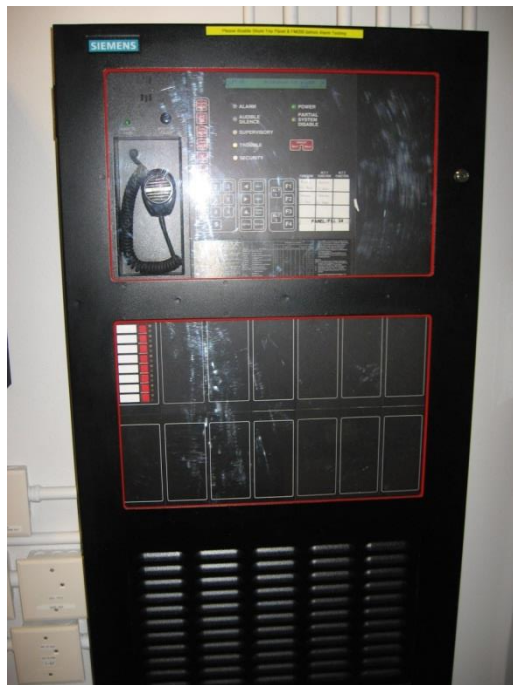
The fire alarm panel for the voice alarm system in suite 121
