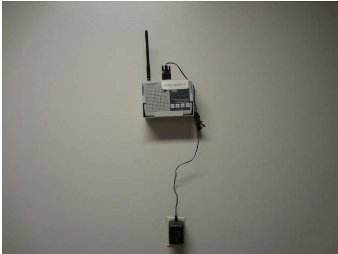
One of 30 Tone Alert Radio (TAR) units in building 910
