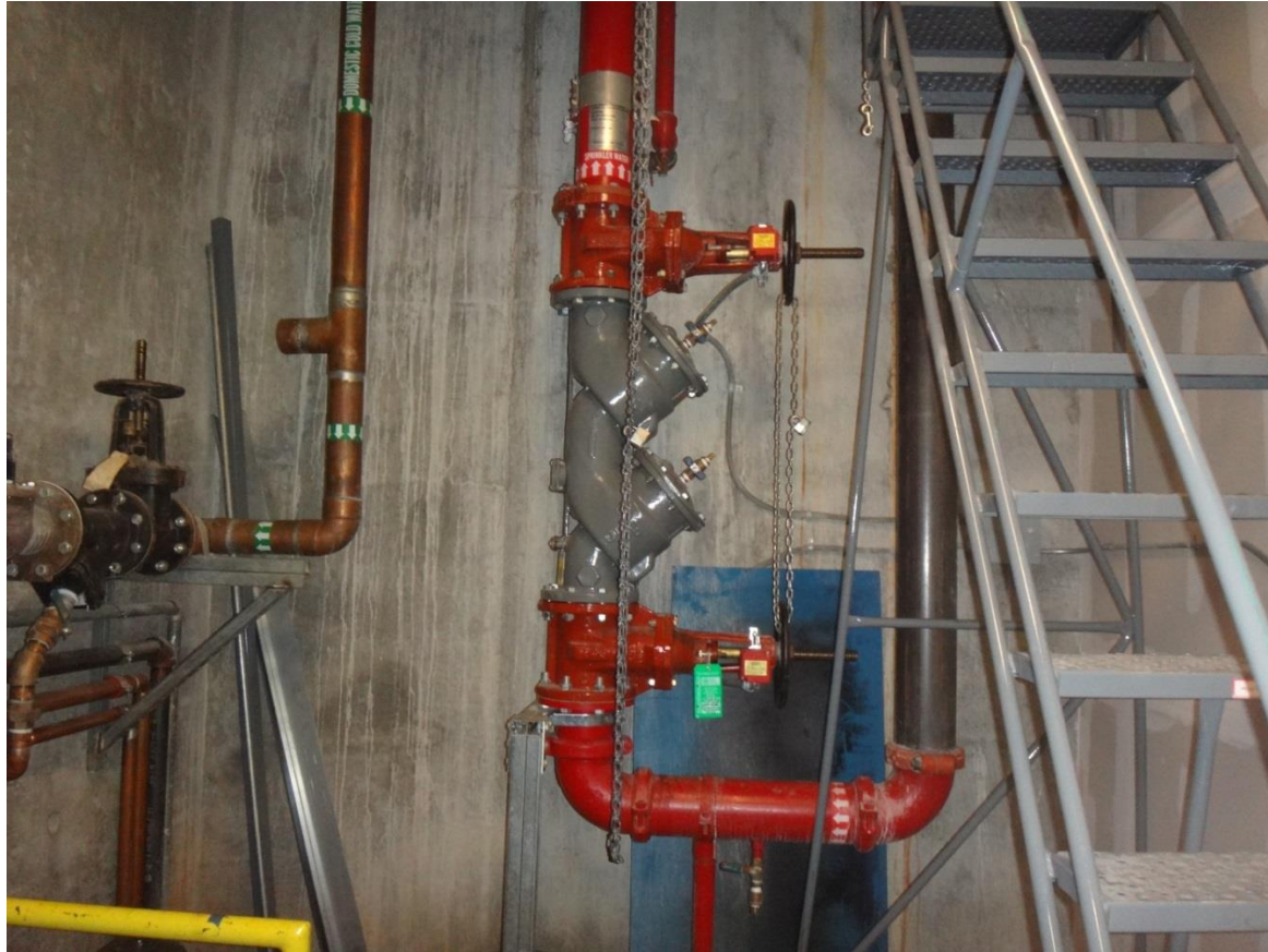
Smaller of the two risers, located in the West end of the building.
