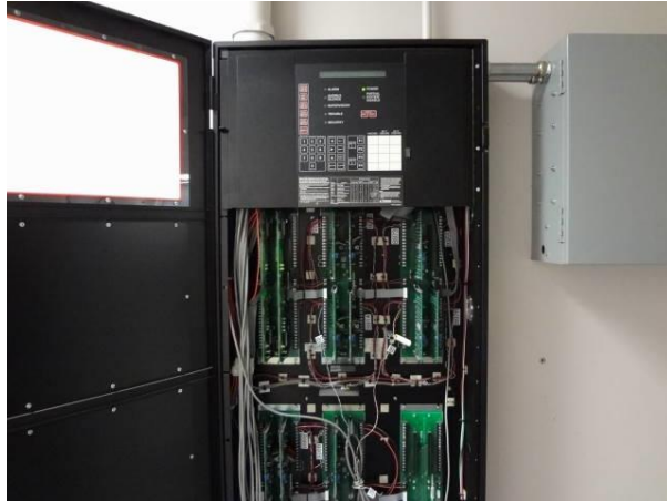
Main fire alarm panel located in the basement
