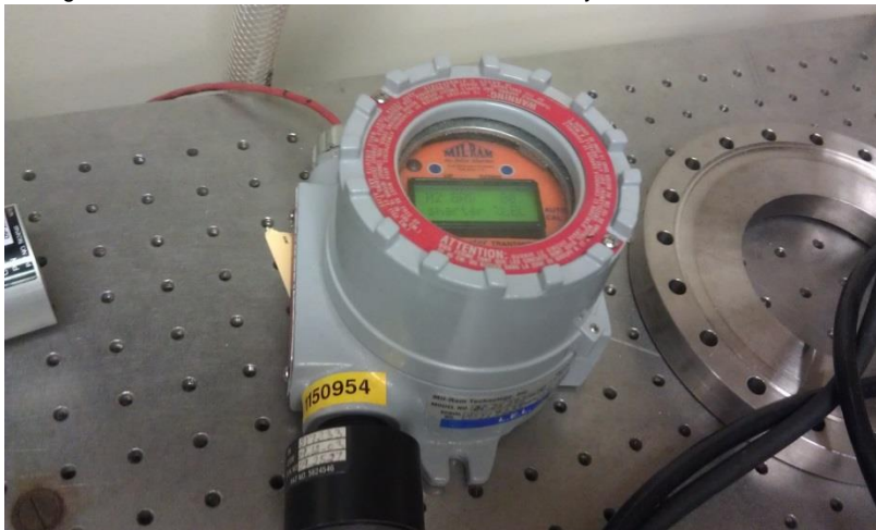
A flammable gas detector in building 910
