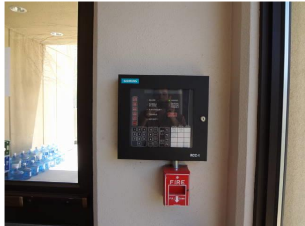
Supplementary fire alarm panel on the first floor
