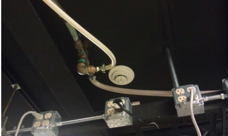
Ceiling Mounted smoke detector in a laser laboratory environment
