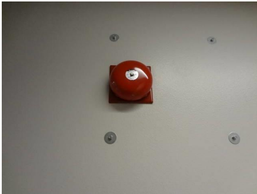
A wall mounted fire alarm bell in building 910.
