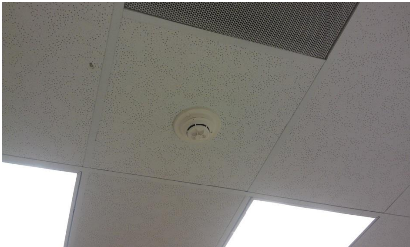
Ceiling mounted ionization smoke detector in a laboratory
