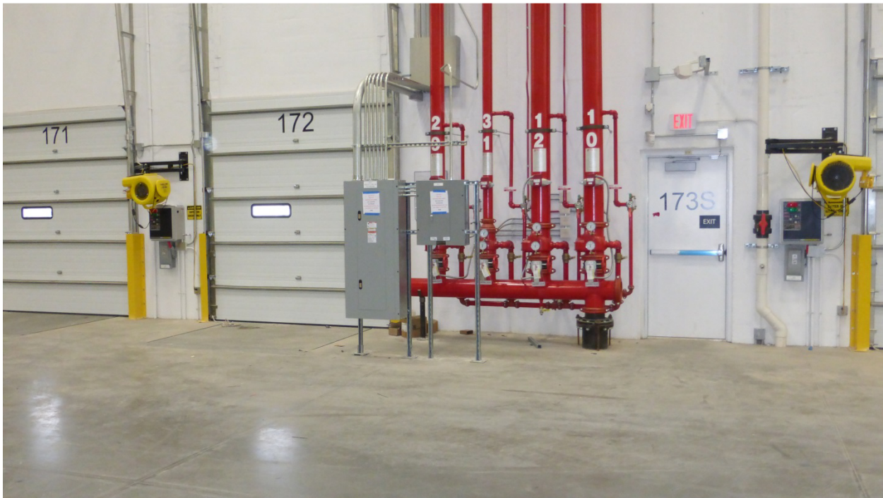
Figure 6: Representative Photo of a More Typical Riser Installation
