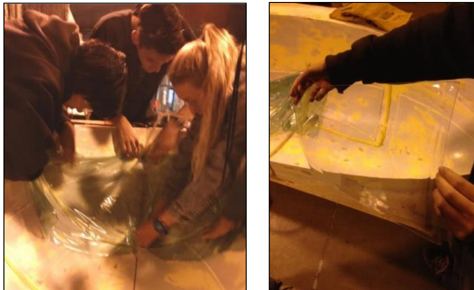
Figure 109. (Right) Team members sealing the vacuum bag during the front windshield heat shaping. The two top molds were bonded together to allow seamless heat-forming. (Left) The finished side windshield.
