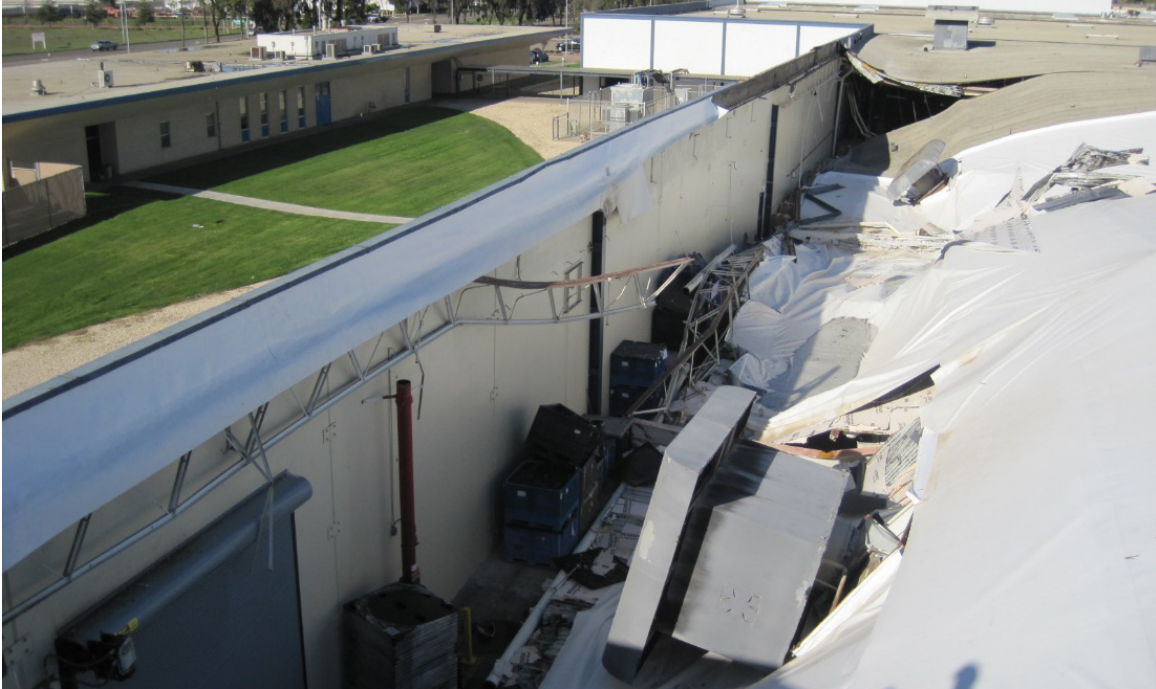
Figure 1 - Excessive rainwater load causes a steel roof structure to collapse. (Source: John Lawson)
