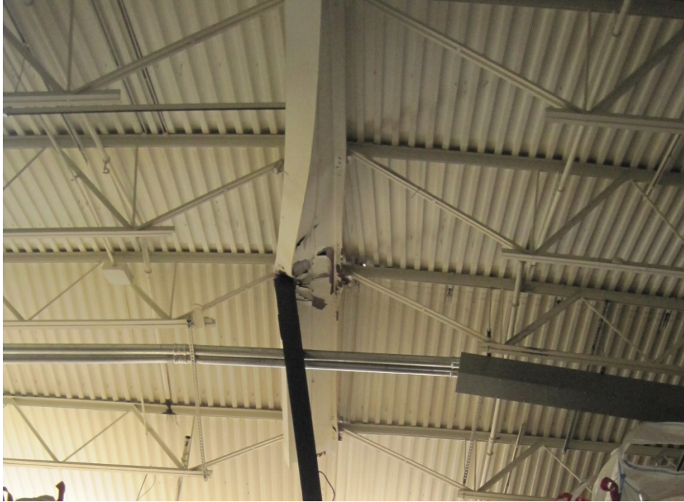
Figure 6 – Girder to Column Stability Failure (Source: Michael Parolini)
