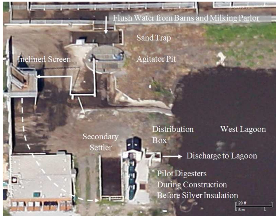
Figure 3.2 Primary flush water treatment area. Pilot digesters under construction here. The distribution box was the source of influent flush water for the digester systems.
