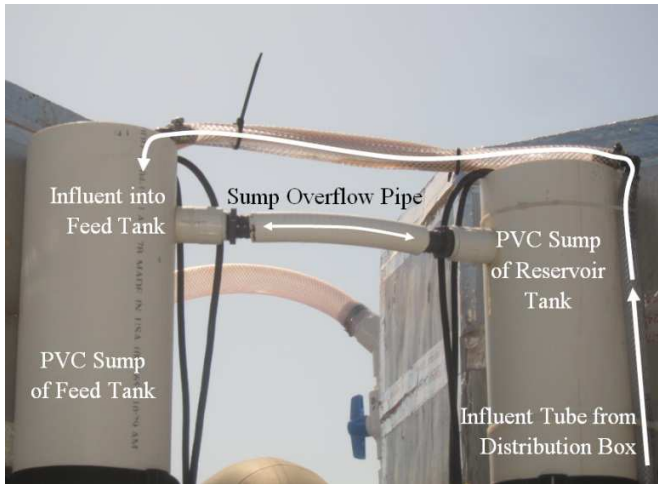
Figure 3.7: Influent flush water tubing with sumps and sump overflow pipe.
