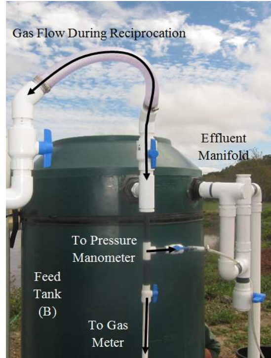
Figure 3.10: Biogas manifold. Reciprocation flow directions, manometer and pipe to gas meter shown. Photo taken before placement of insulation.
