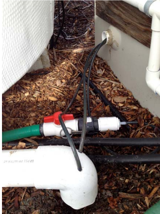
Figure 3.4: Effluent from both 2-day Round 1 ponds were mixed in a 3" PVC manifold connected to the drains of both ponds. This mixing was necessary so that the tube settlers received the same influent. The combined Round 1 effluent was pumped out of the PVC manifold using peristaltic pumps and tubing inserted into the end of the pipe. The pumps moved the Round 1 effluent to two tube settlers. Effluent from the 3-day Round 1 pond was collected in the green tube connected to the pond drain.
