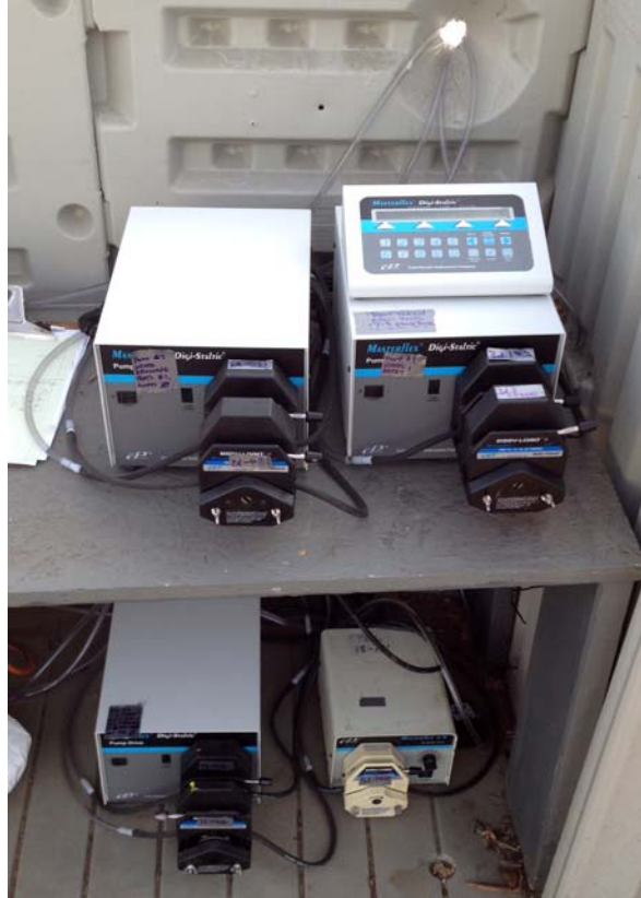
Figure 3.5: Peristaltic pumps in the pump house. The pumps on the top shelf pumped primary effluent to the Round 1 ponds. The pumps on the bottom shelf pumped Round 1 pond effluent to the tube settlers
