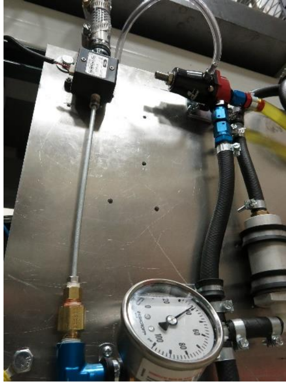
Figure 27. Upstream plumbing of flow meter
