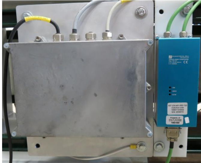
Figure 6. Power Supply and Torque/Speed Conditioner Mounted
