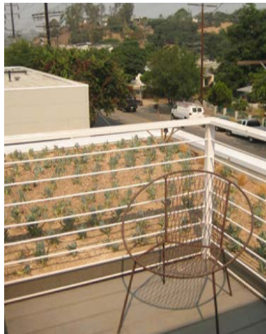
A green roof helps absorb runoff, reduces the heat island effect, and provides an attractive amenity for residents.
