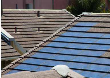
The Gatsby Homes integrate photovoltaic panels into its roof for enhanced energy efficiency.
