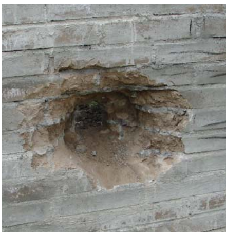
Figure 13: Double wythe wall and penetration by a chipping action of the hammer head, front face
