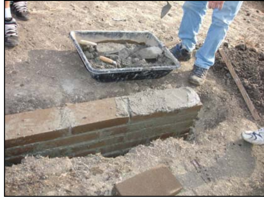
Figure 5: Brick wall laid directly on ground starting 5 course below grade
