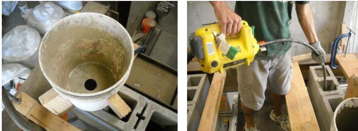
Figure 8: (a) Grout Funnel Leading into One Grout Column and (b) Mechanical Vibration
