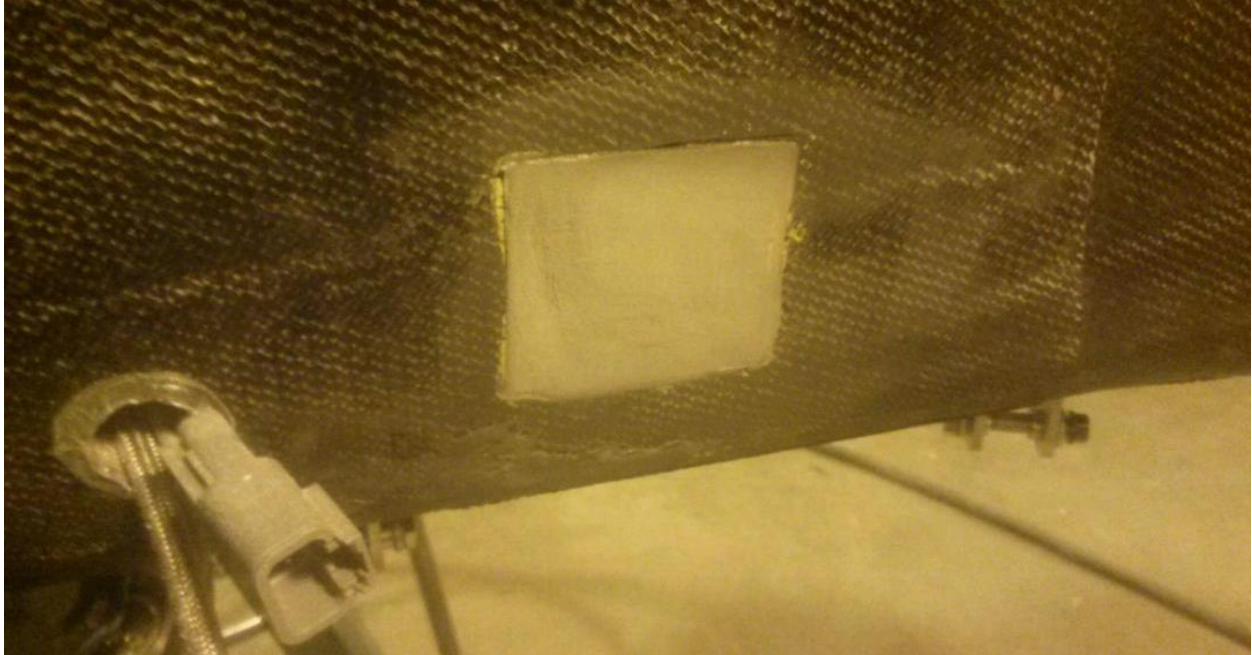
Figure S5. 0.750" thick end-grain balsa wood was cut into a 2"x 2" square and test fit in the cavity. Next it was scuffed with sandpaper and wiped clean with a new towel.
