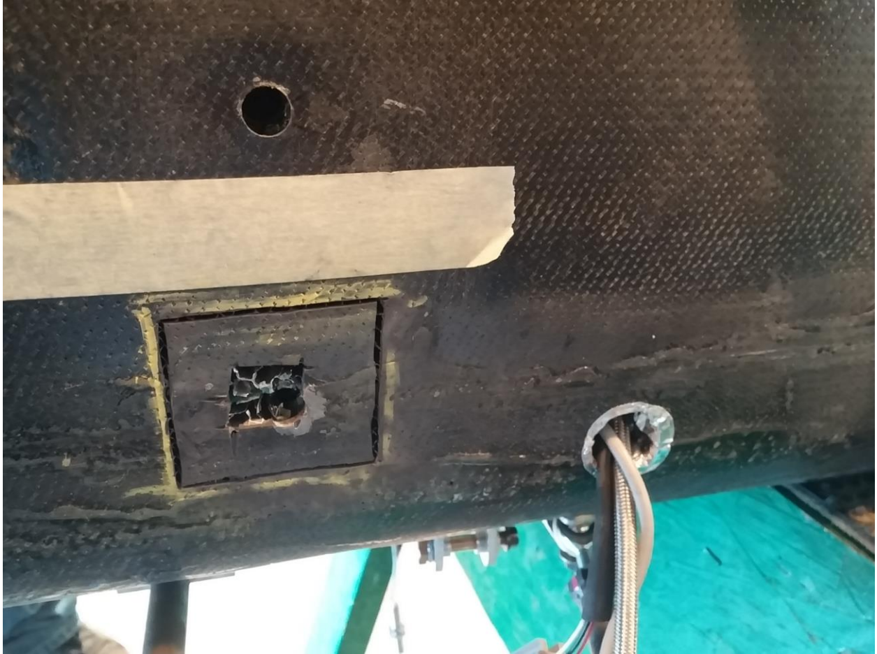
Figure S2. When full core failure was observed, the repair began and a 2" x 2" square was cut using a rotary tool and cutoff wheel.
