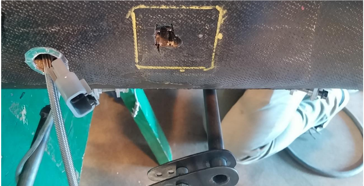
Figure S1. First a small opening was made with a rotary tool to inspect the core for damage.
