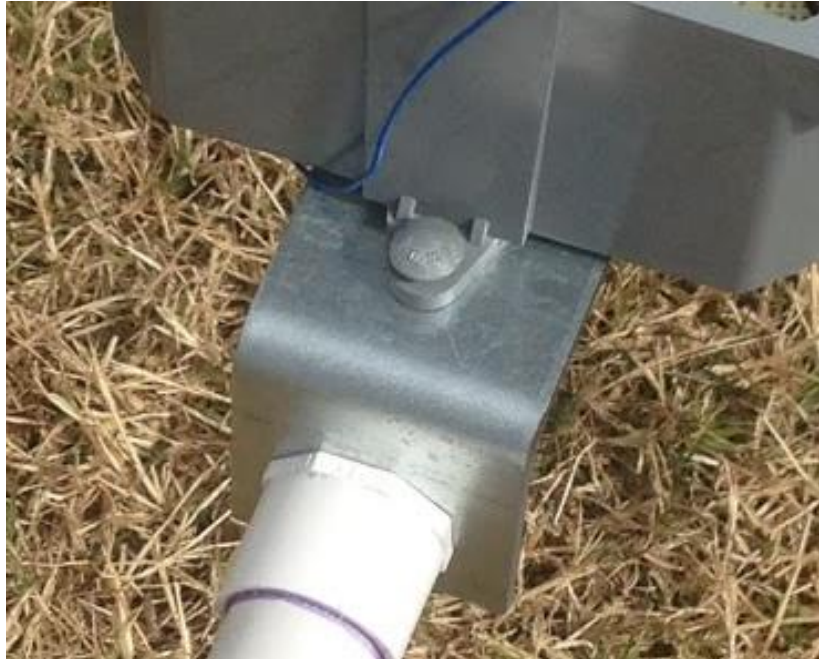
Figure 29: Close up, top view of bracket, bolt, and box connection.
