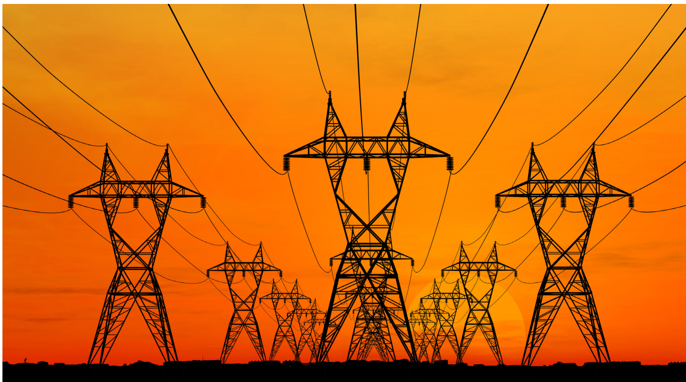
Figure 2.10: Transmission lines. Sourced from Brown (2012)
