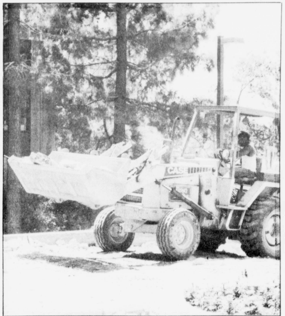
The walkway between the University Union and the Administration building was torn up Wednesday / Photo by Lawrence Rodenborn
