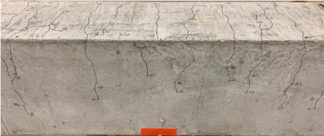
Figure 4.40: Typical Flexural Cracking within Confined Splice Region (C3/60-40-5-200)
