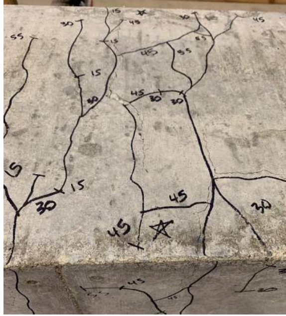
Figure 4.59: Longitudinal Crack Branching (C3/60-50-5-200)
