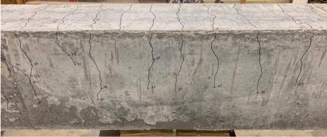
Figure 4.39: Typical Flexural Cracking within Unconfined Splice Region (U-60-10)
