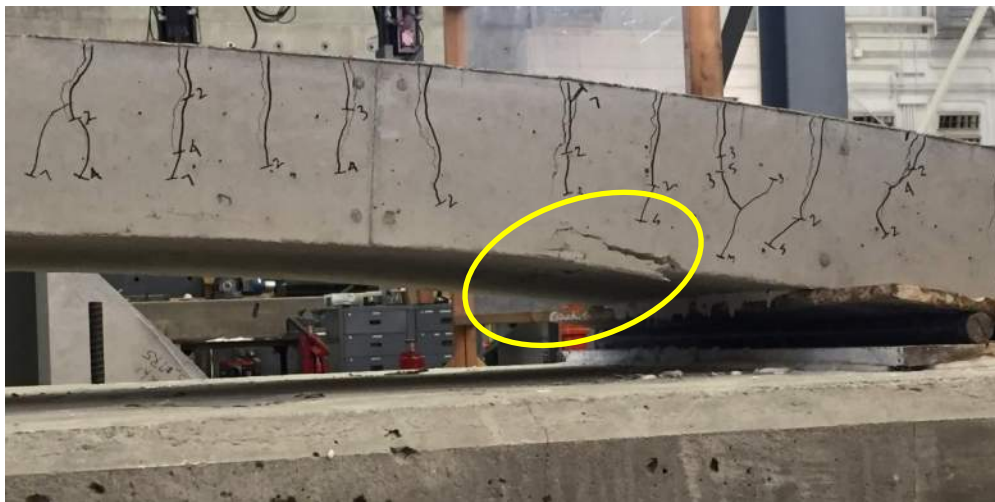
Figure 3.50: Initiation of S-80-5 Failure – East Elevation
