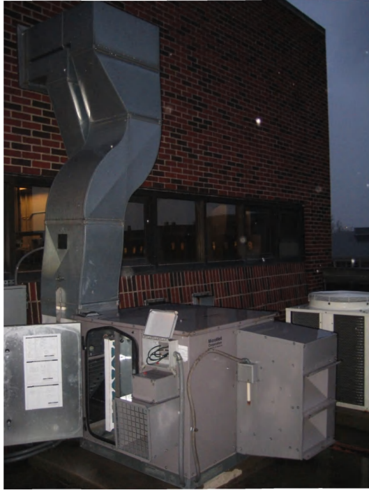
Figure 2 – Supply air duct maintenance panel
