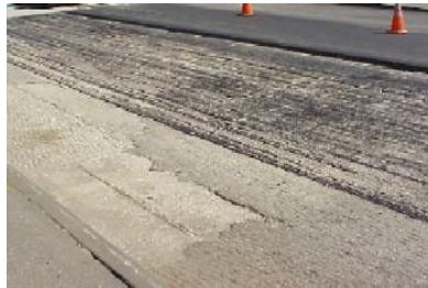
Gambar 2.6 Peyempotran Tack coat Buruk (Sumber: http://pavementinteractive.com )
