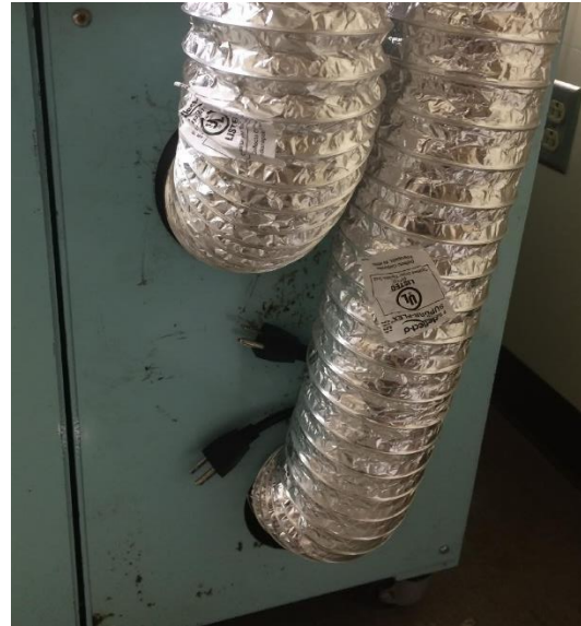
Figure 71: Ducts and 5" holes into cabinet
