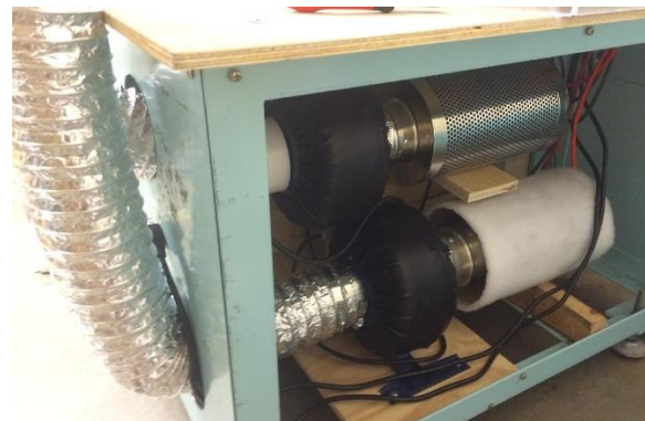
Figure 72: Fans mounted inside table
