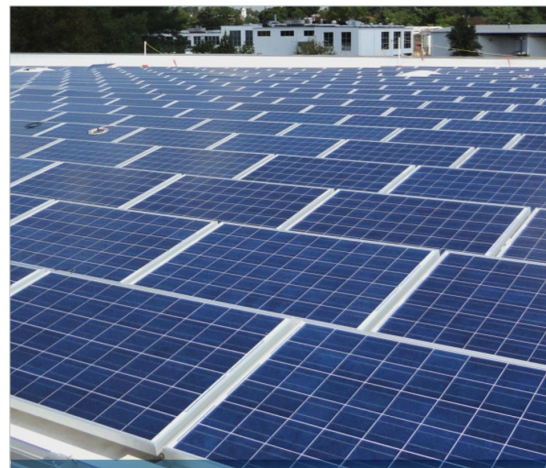
Figure 2.10: Roof top-mounted solar panels conserve electricity, thus preserving natural resources
