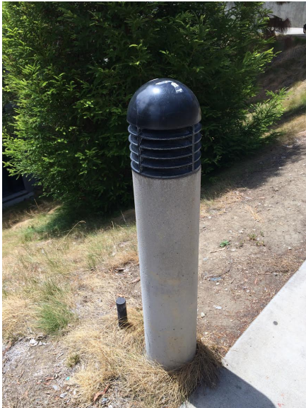
Figure 85: Dysfunctional lighting fixture
