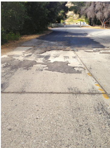
Figure 25: Damaged street area near Cuesta Park
