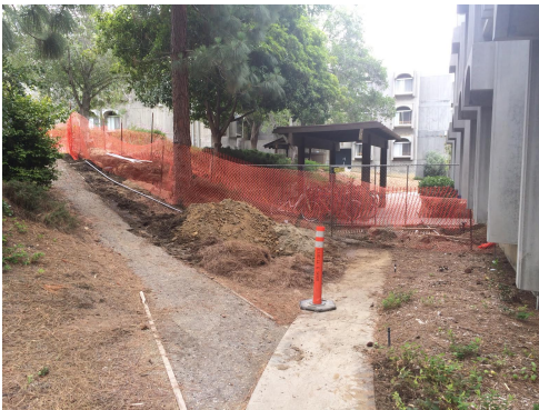
Figure 73: Ugly construction area behind dorm
