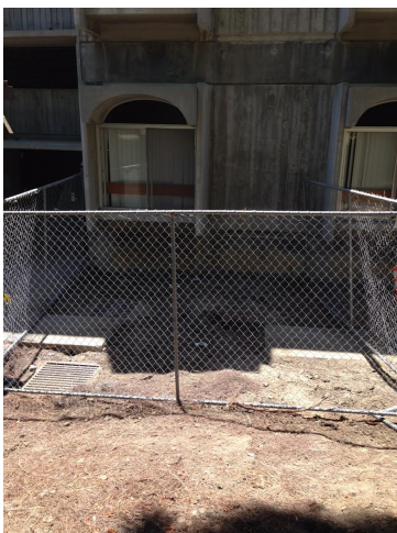
Figure 65: Ugly construction area
