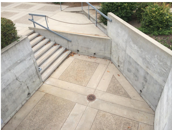
Figure 95: Underutilized cement enclosure
