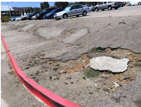
Figure 89: Crumbling asphalt groundcover
