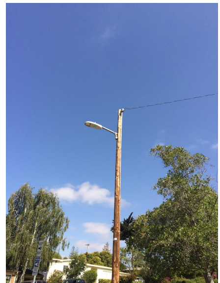
Figure 44: Light fixture in Buena Vista Park
