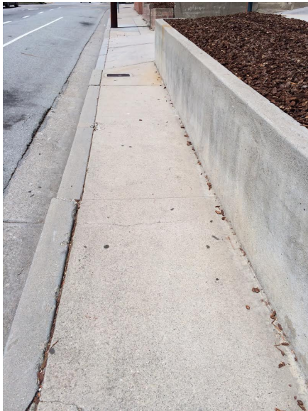
Figure 43: Narrow sidewalk on Grand Avenue
