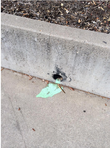
Figure 93: Green substance coming out of drainage pipe
