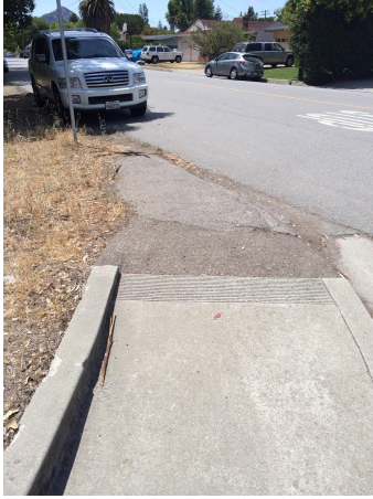
Figure 51: Abrupt end of sidewalk
