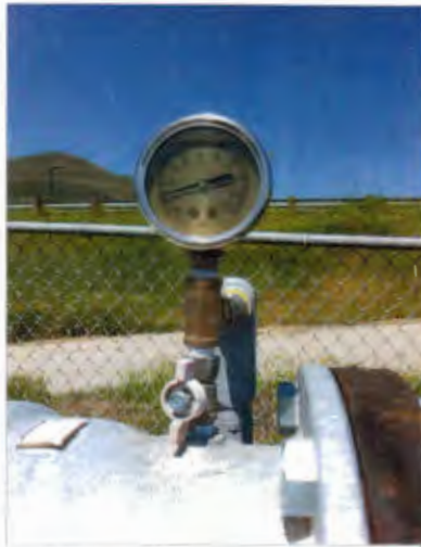
Figure 13: Pressure Gauge for Shepard Reservoir
