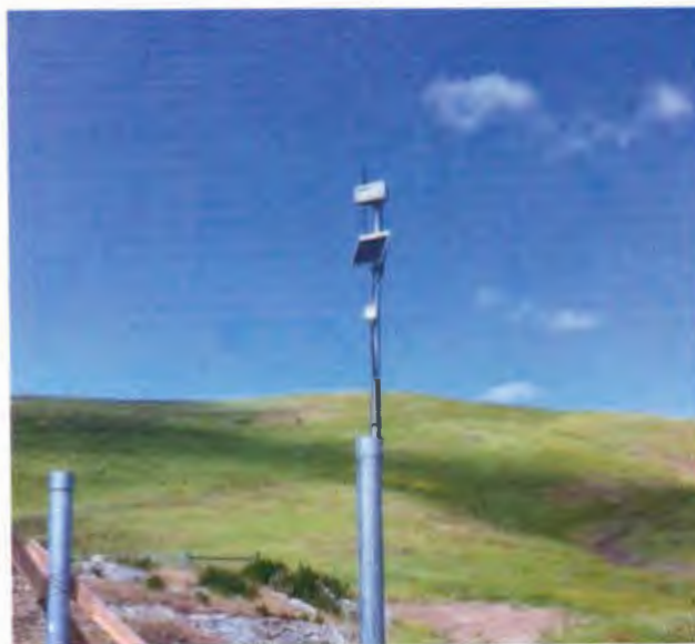
Figure 29: Complete Nelson Reservoir Adcon Telemetry Station
