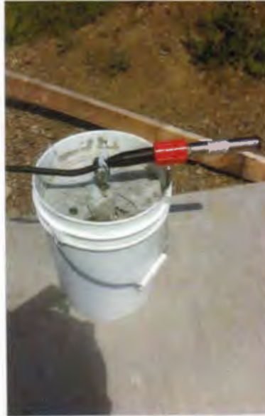
Figure 25: Water level sensor secured to weight
