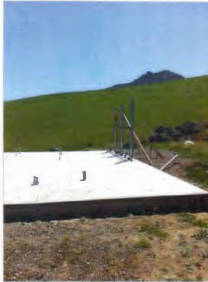
Figure 27: Pump pad at Nelson Reservoir
