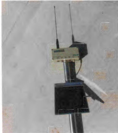
Figure 23: RTU and Solar Panel Assembly
