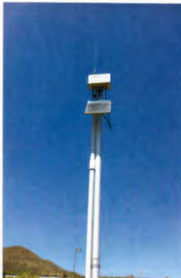
Figure 15: Adcon Telemetry Station at Sports Complex
