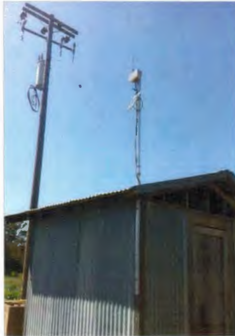
Figure 7: Field 25 RTU on pump house
