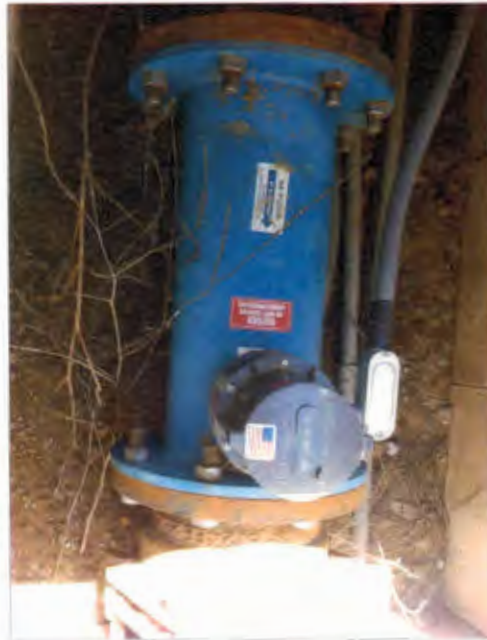
Figure 14: One flow meter at Sports Complex
