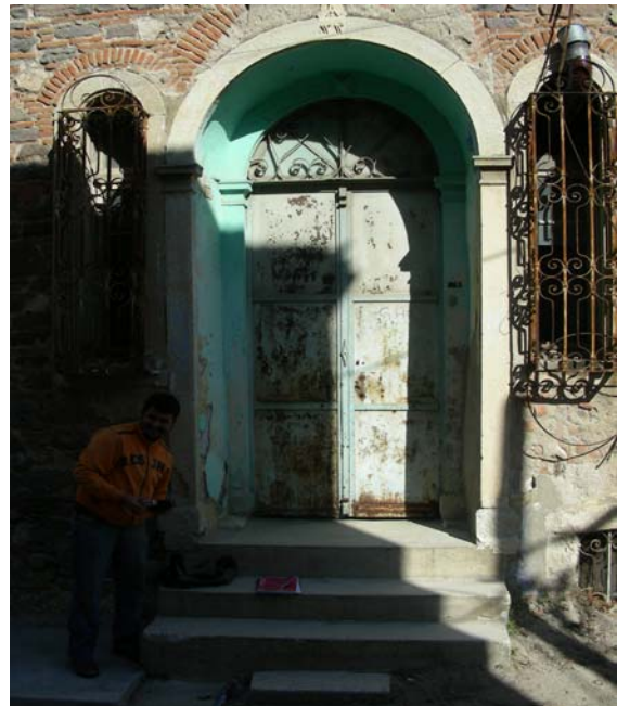
Figure 3.33. Two winged, iron door (404th Street No. 9-11) Identical twin doors for twin buildings; there is a stone relief carved above the doorpost.
