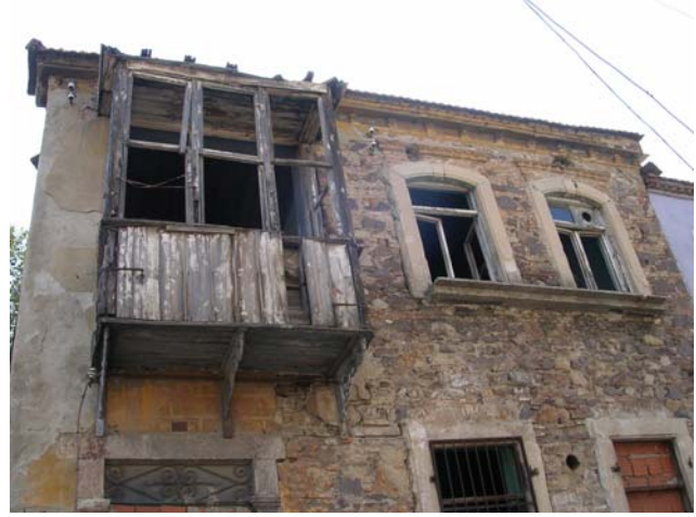
Figure 4.9 Ruined building on 403 Street No. 28
