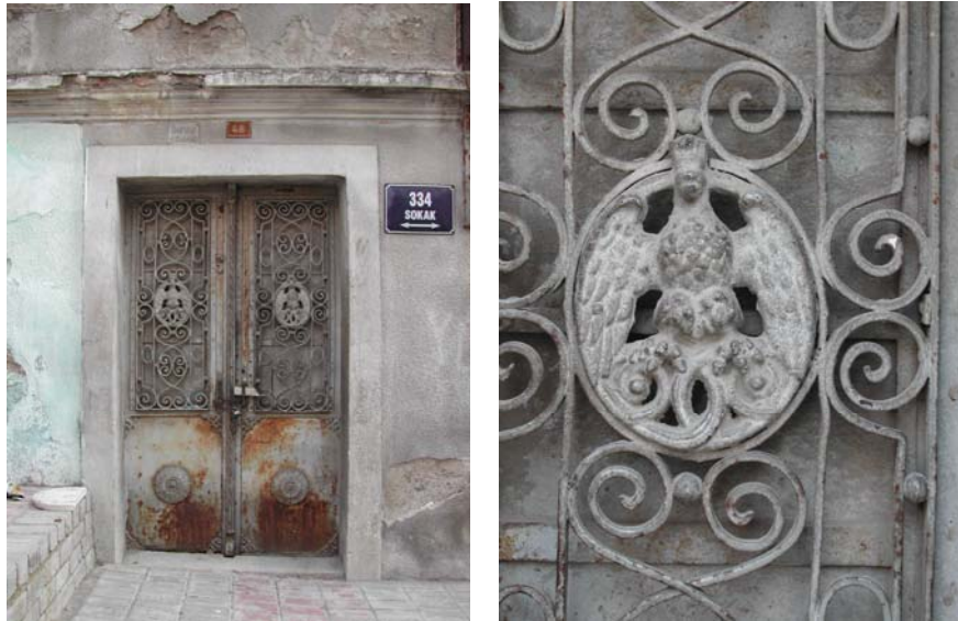
Figure 3.34. The eagle motive on the two winged iron door (334th Street No. 46)
