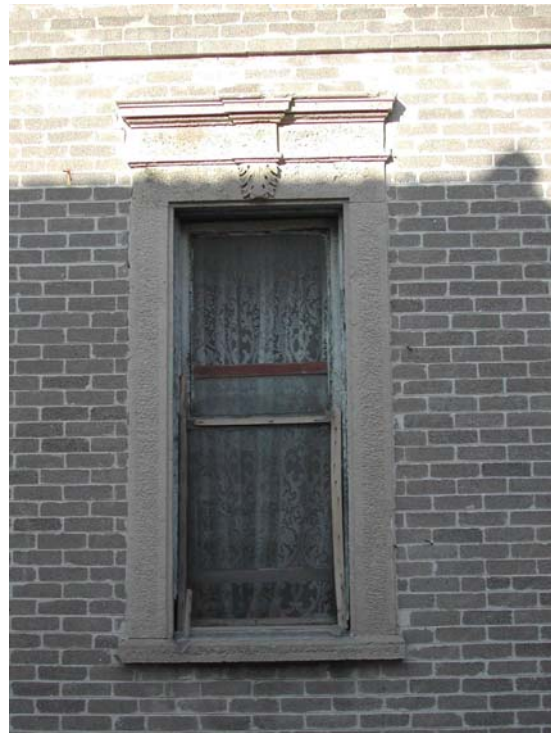
Figure 3.38. Wooden guillotine window surrounded by jambs and decorated with a relief carved on the key stone (384th Street No. 65)
