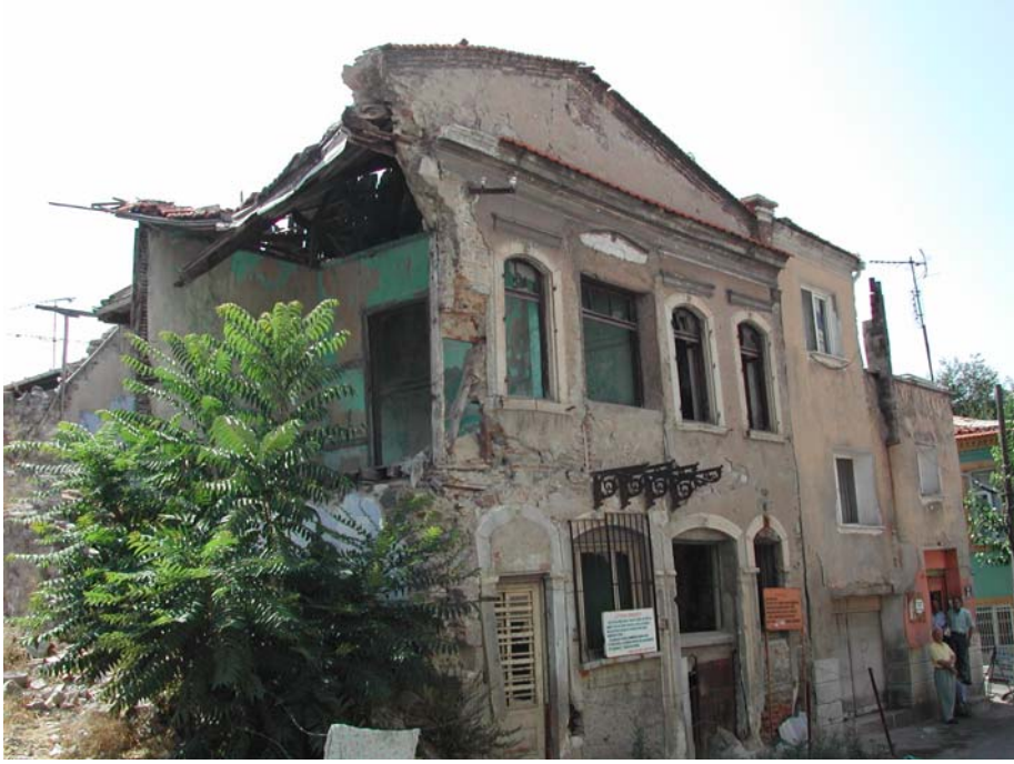
Figure 4.12 Ruined building at 384th Street No. 22
