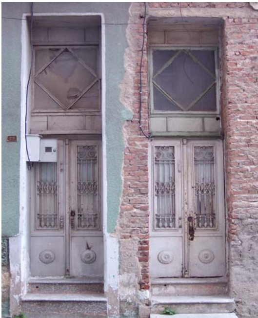
Figure 3.32. Two winged, iron door (404th Street No. 27-29) Identical twin doors for twin buildings
