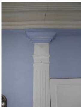
Figure 3.13. First floor, next to the room door, 384 Street No. 65
