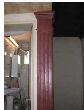
Figure 3.15. First floor, next to wc door, Halil Rifat Paşa Street
