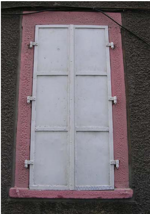
Figure 3.37. Although it is an upper floor window, an iron shutter is used. (S2 zone)
