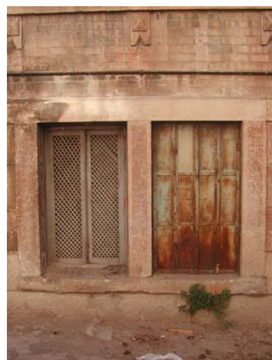
Figure 3.44. A ground floor window opening towards street; a wooden shutter and an iron fence are positioned side by side. (Halil Rıfat Paşa Street)
