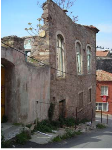
Figure 4.8 Ruined walls belonging to Selimiye Mosque on 404 Street
