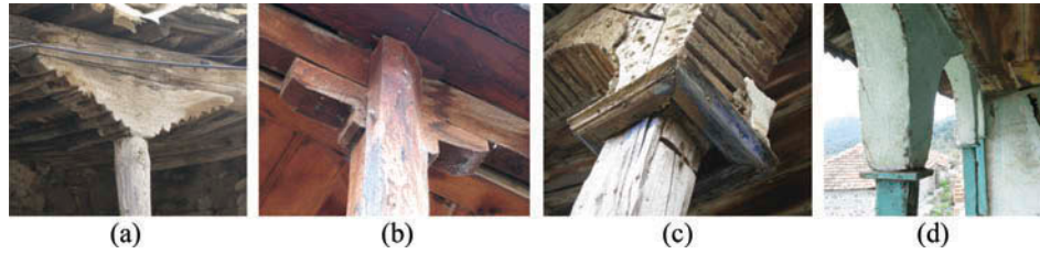
FIG. 21. Timber elements supporting roof-eaves of the sofas (Bergama-Yukarıkırklar): (a) single-piece capital, (b) a double-piece capital, and (c–d) arch imitations with bağdadi technique.
