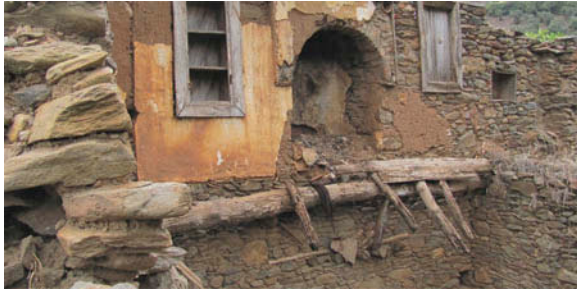
FIG. 18. Floor system of a collapsed house (Beydağ-Alakeçili).
