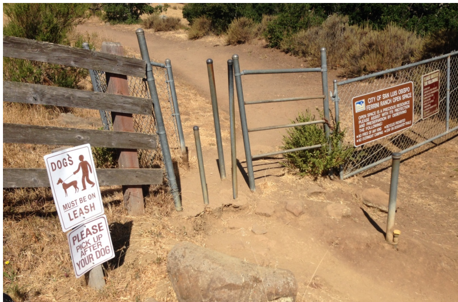
Figure 5: The entrance at the Patricia trailhead is eroded and has several narrow turnstiles.
