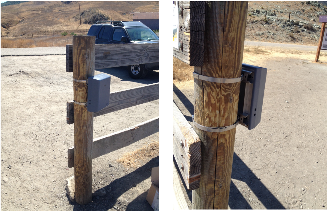
Figure 61: Johnson Ranch Trailhead Eco-counter Installation
