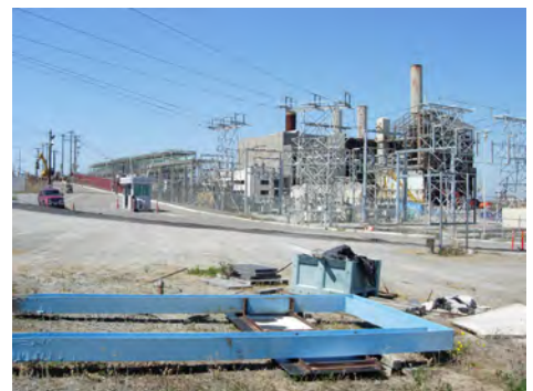
Figure 2.3 Existing PG&E Power Plant Structures Electrical Grid Network in Foreground is Remaining Building Structure in Background is Under De-Construction Process
