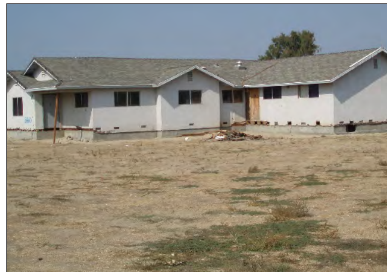
Image XII: Dilapidated parcels consisted of structures showing major structural damage. Structure also appeared to be uninhabitable due to safety concerns and substandard living conditions.
