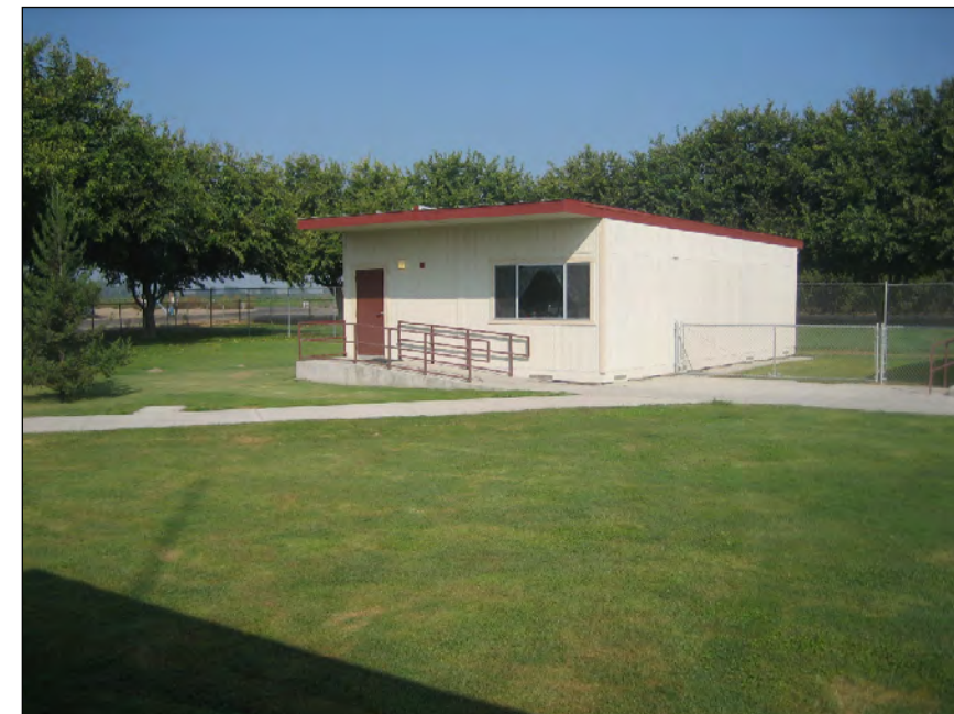
Image II: Just one of the bungalow-type structures of the school. To serve the community in the future, improvements would have to be made.
