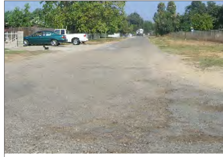
Image XVII: Potholes and uneven surface conditions riddle most streets within the residential neighborhoods.
