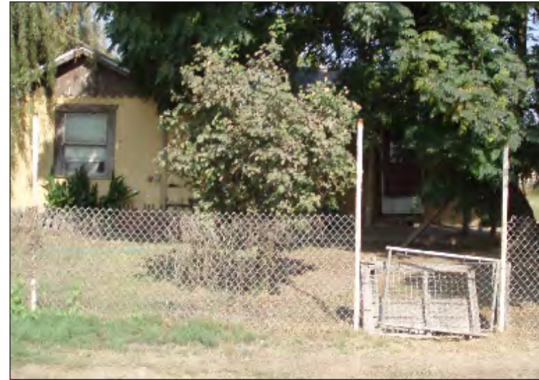
Image XI: Poor parcels consisted of structures that appeared to be in bad condition, yet still habitable. Some minor structural damage was apparent, and extensive maintenance was needed.
