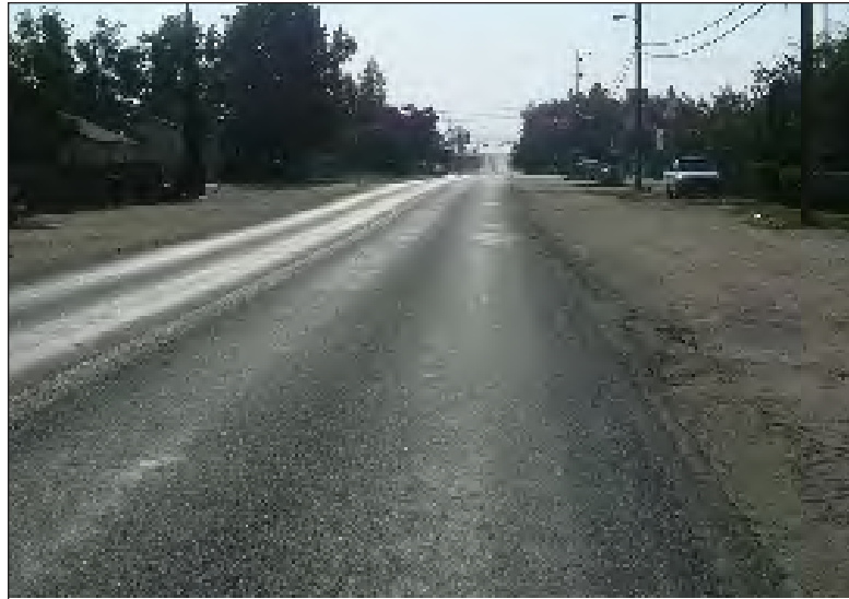
Image XV: Merritt Drive is both poorly surfaced (truck traffic has warped the road's surface) and unsafe for pedestrians walking alongside the road.
