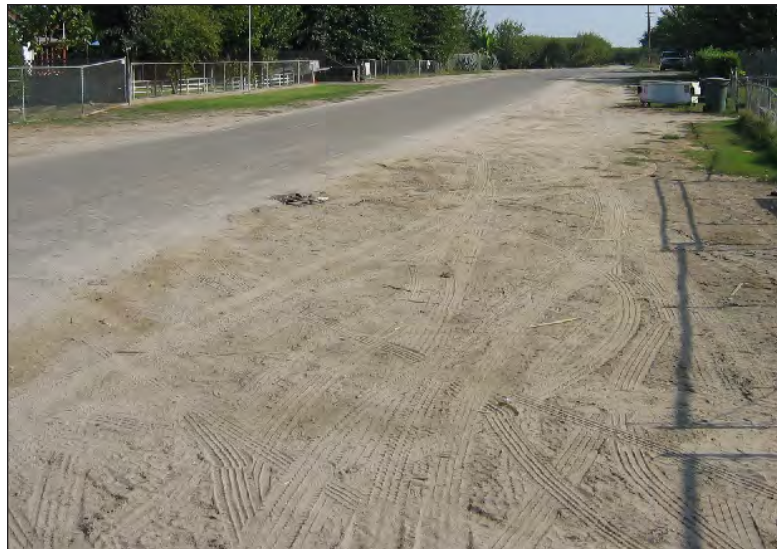
Image XVI: Often roads within this community have no drainage measures or good road shelves.
