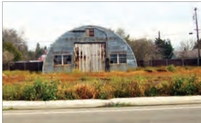
5: Across from the high school, this old structure has potential cultural significance for reuse.
