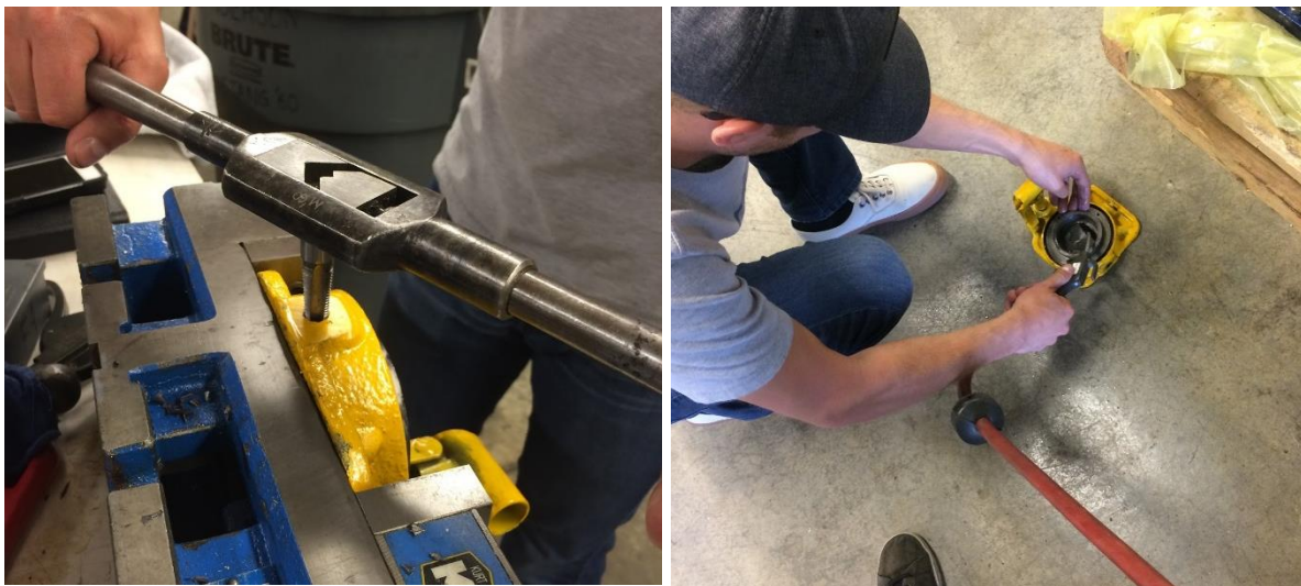
Figure 34. (Left) Cutting \frac{1}{4} " NPT threads for hydraulic fittings. (Right) Cleaning shavings from jack with compressed air.
