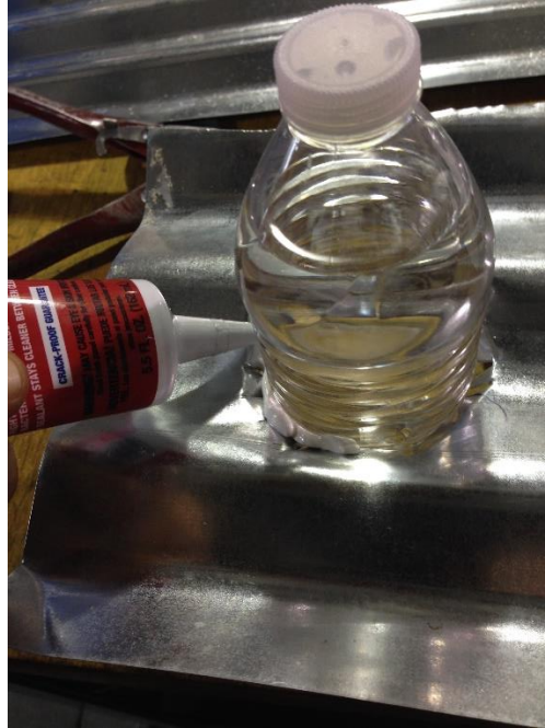
Figure 14. Caulk is applied to create a watertight seal and secure the water bottle light in the roof section
