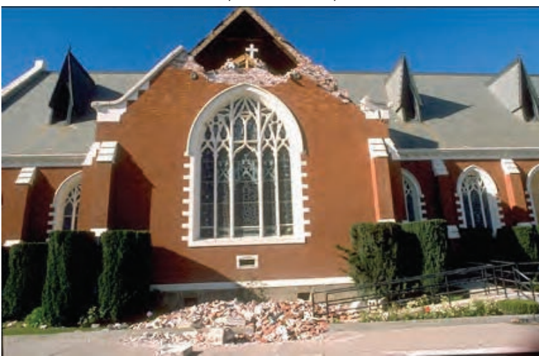
Figure 1: Damage to St. Patrick's Church in downtown Watsonville after the Loma Prieta Earthquake. (Robert A. Eplett/ CAL EMA)
