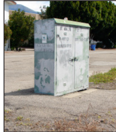
Source: Photo, April 17, 2012 Attempt to remove graffiti from utility box on Railroad Avenue.
