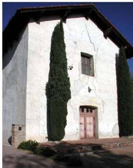
Figure F-5: Mission San Miguel Church taken a few months before the devastating earthquake
