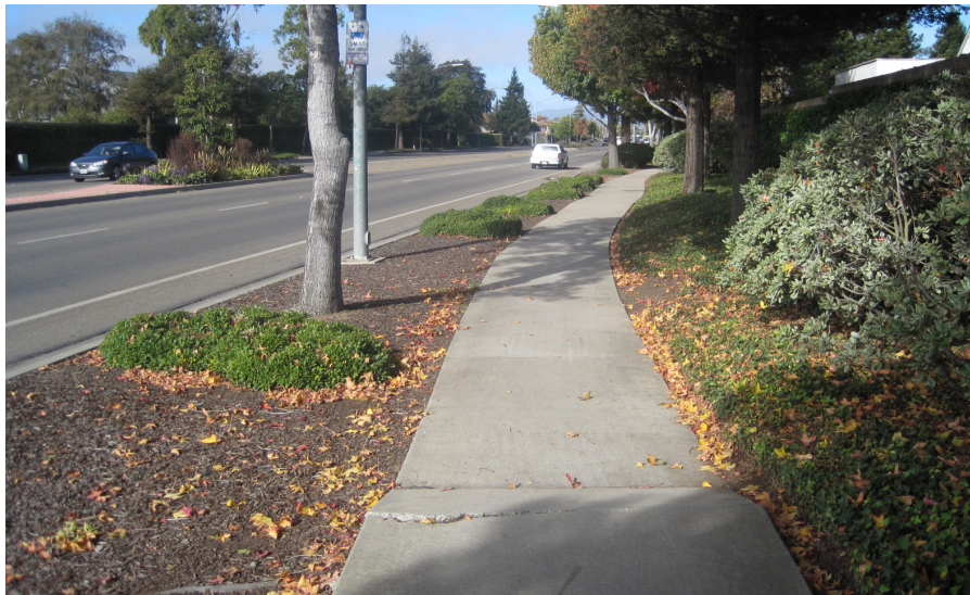
Figure 10: Miller at Battles stop with uneven sidewalk.
