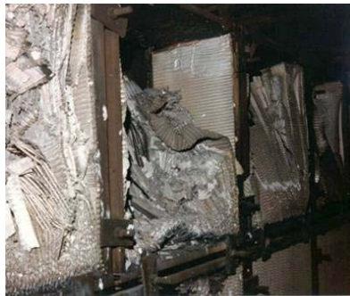
Figure 2: 1969 fire filter damage
