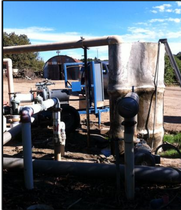
Image of Filter, Pump and Concrete Standpipe at Underwood Orchard
