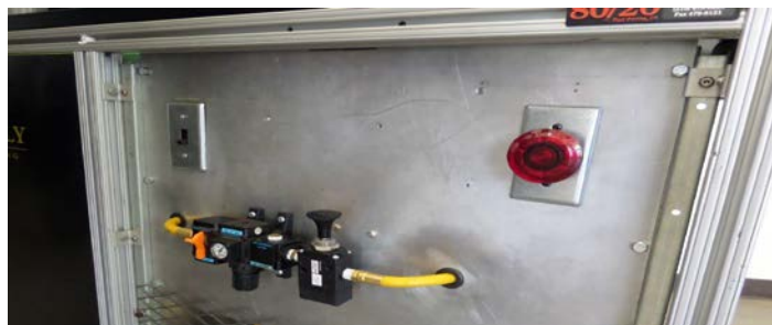
Figure 6. Control Panel Features
