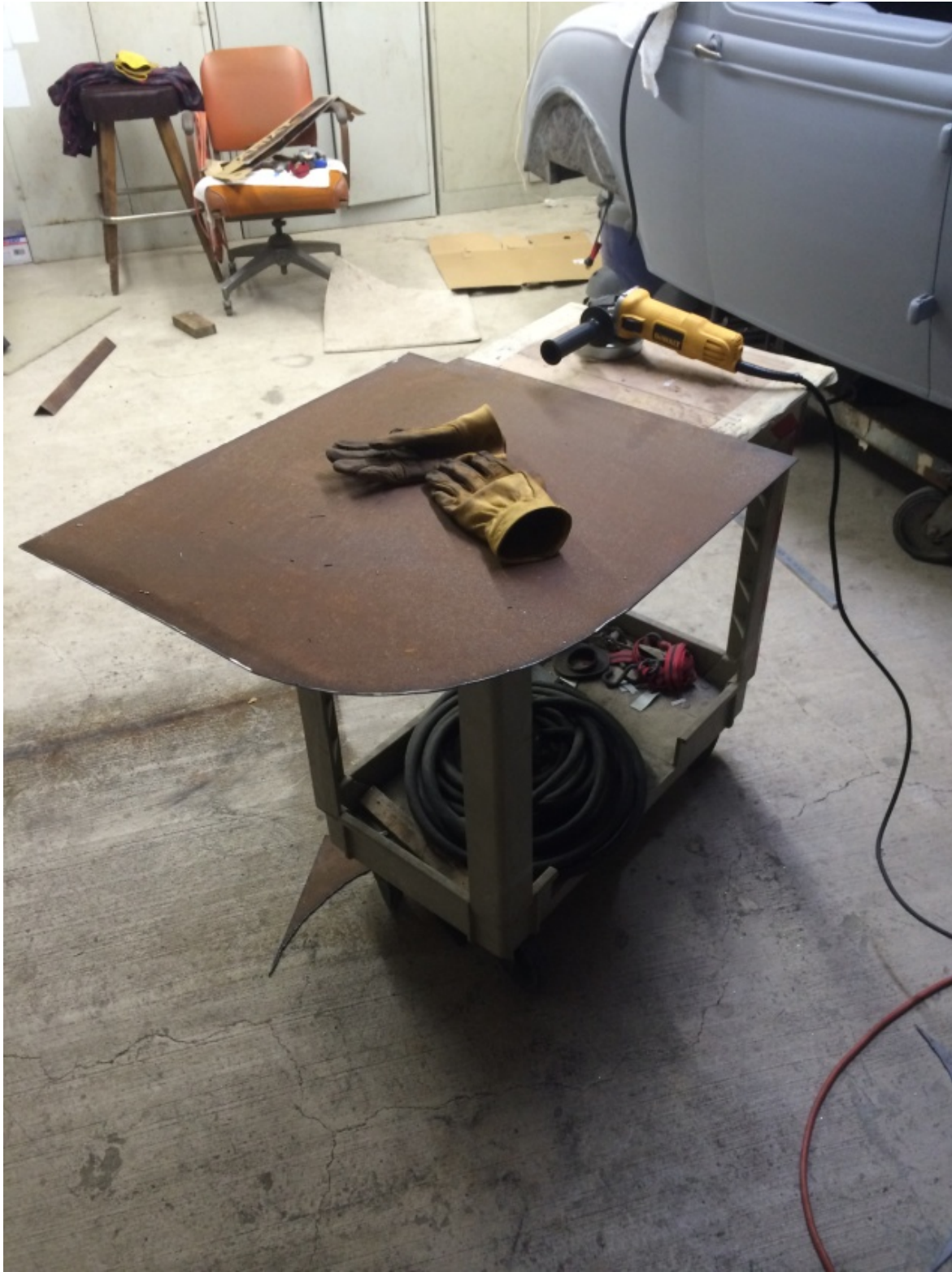
10 Gauge sheet metal cut with a plasma torch to fill in the half doors on the trailer.
