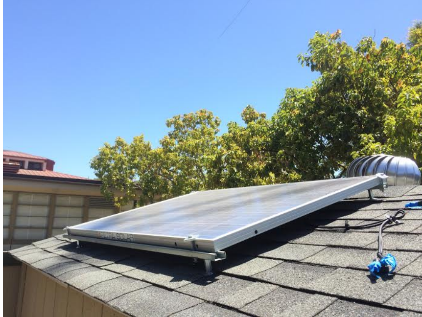
Figure 4-3: Solar Panel Mounted on the roof of the DC House
