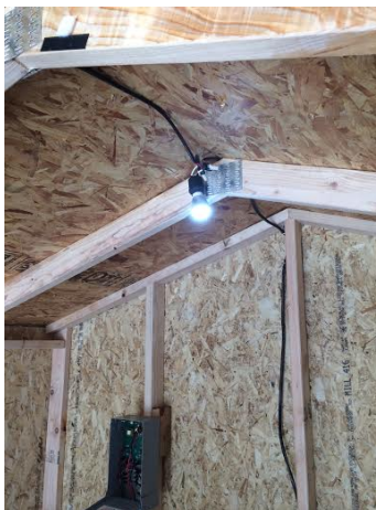
Figure 5-7: Lighting Circuit Powered ON
