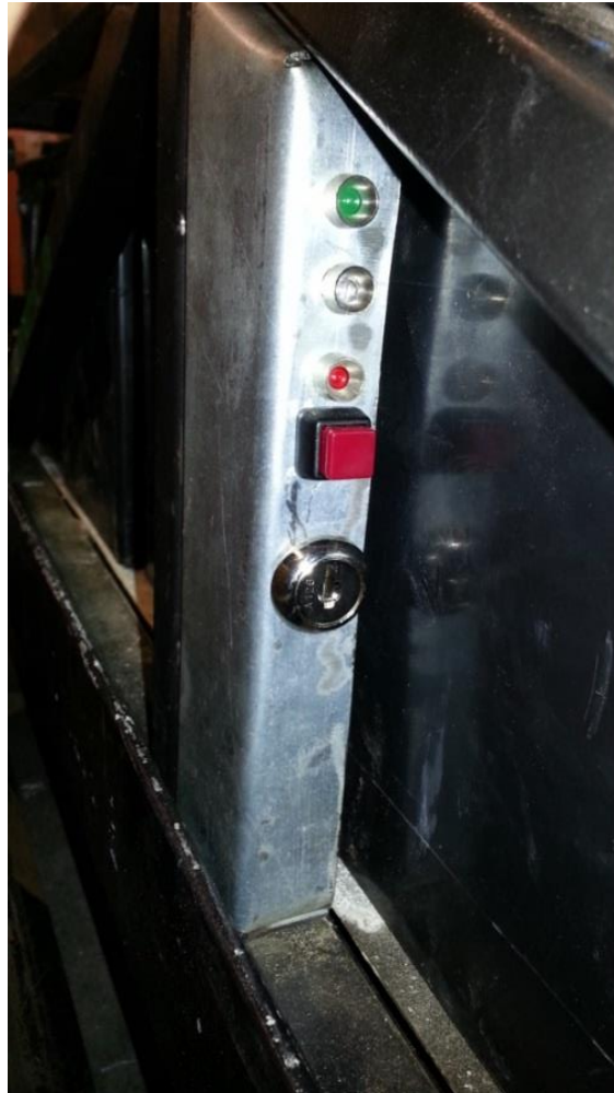
Figure 31: Battery pack status and manual control panel
