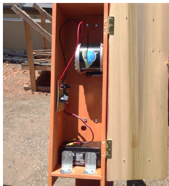
Figure 4-6: Compartment box covering all the electrical components in the system
