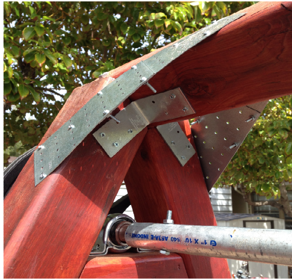
Figure 4-5: Metal plates added for stability at the top corners of the structure
