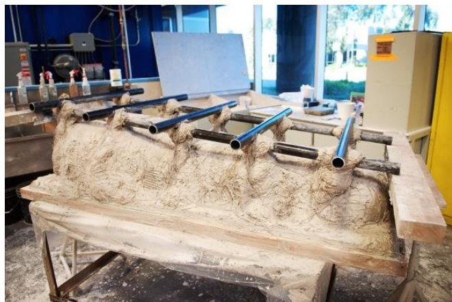
Figure 9.6 - The main support structure added to the mold. Hemp, plaster and a tubular steel framework.
