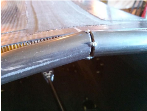
Figure 9.54 - The front roll hoop fit into the tub and tack welded into place.
