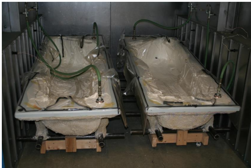
Figure 9.25 - The parts under vacuum and ready for the cure cycle to start.
