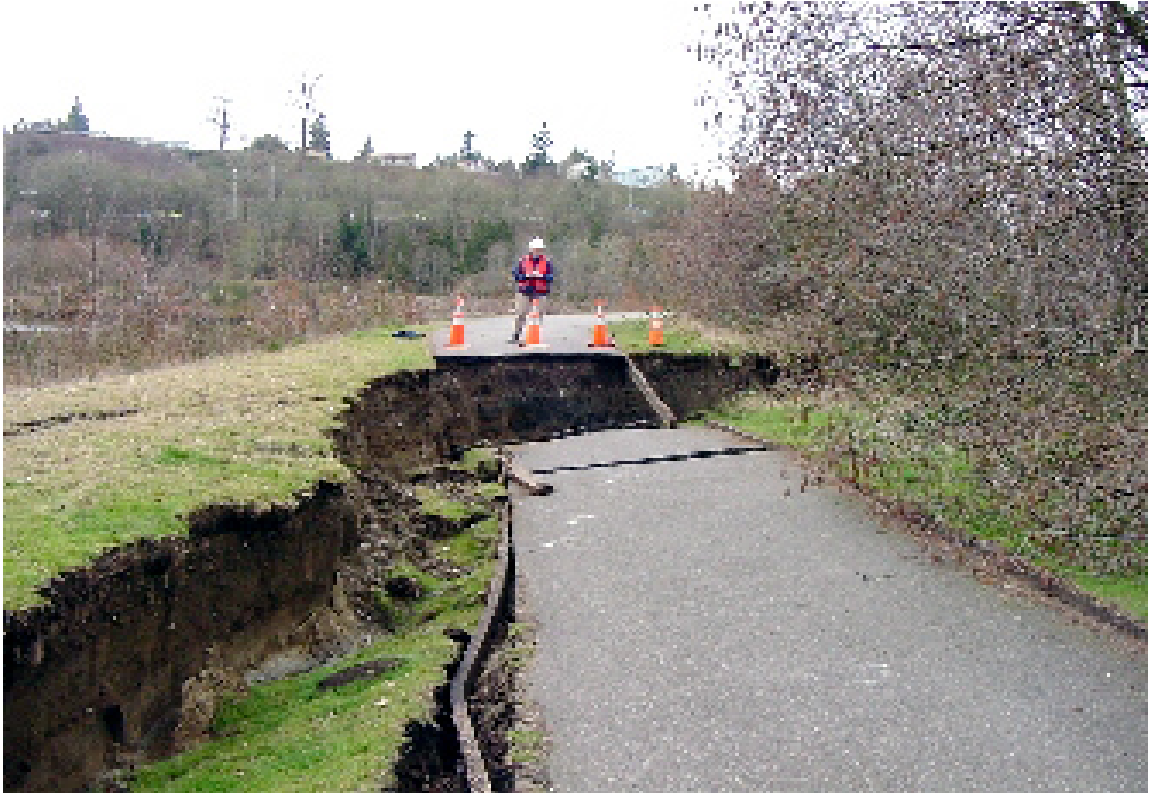
Figure 3. Lateral spread damage caused by Nisqually Earthquake (2001). Damage located at the Capitol Interpretive Center, Deschutes Parkway, Olympia, Washington. Photo downloaded from the PEER Report “ Some Observations of Geotechnical Aspects of the February 28, 2001, Nisqually Earthquake in Olympia, South Seattle, and Tacoma, Washington ”:
