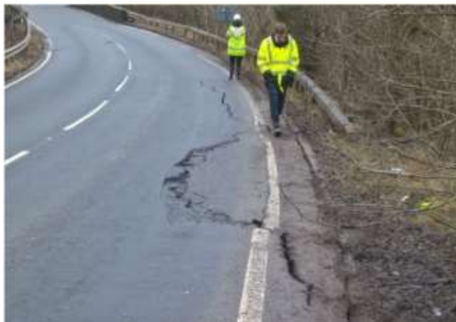
Figure 1.1. Cracking appears on the embankment shoulder in A801 Avon Gorge road, UK.
